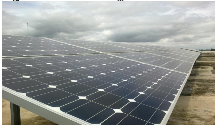
Figure 1: Details of Solar panels
